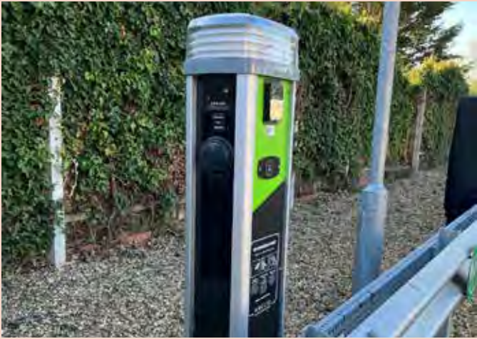
EV charging point
